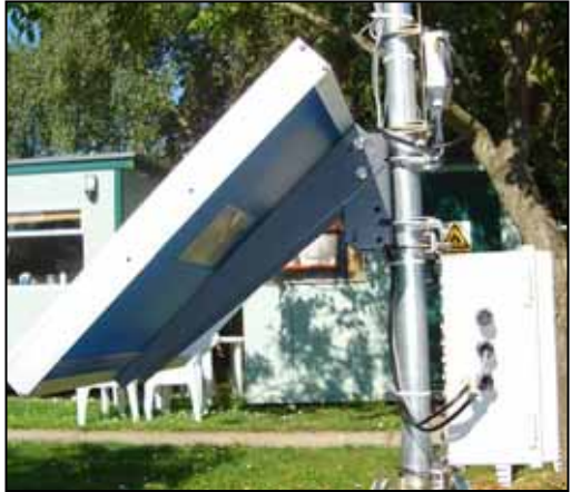
Showing a GP1 logger (at top), solar panel and GSM Modem Box, each fixed to a post using U-bolts and mounting brackets.
