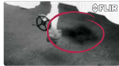
Captured gas leak from production site.
